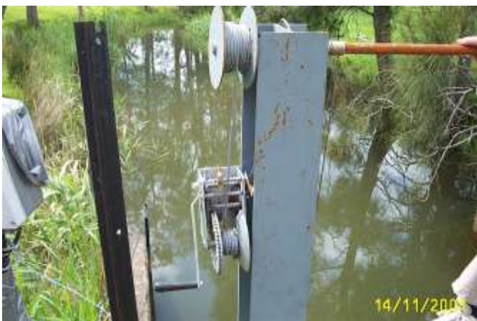
Manual winch to raise and lower gate. Next stage is to have gate automatically controlled.
