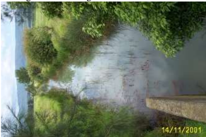
look west from normal floodgate. Leakage of saline water with acidic water turns water milky. Ph about 4-5.
